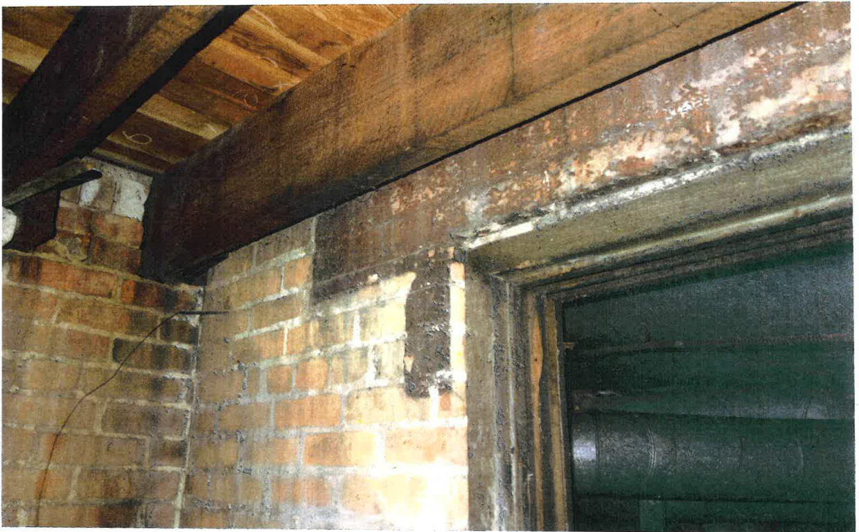
"Ghost" outlines of steps from the now-missing original service stair, surviving in the paint of the basement wall under the rear gallery (center of photo)
